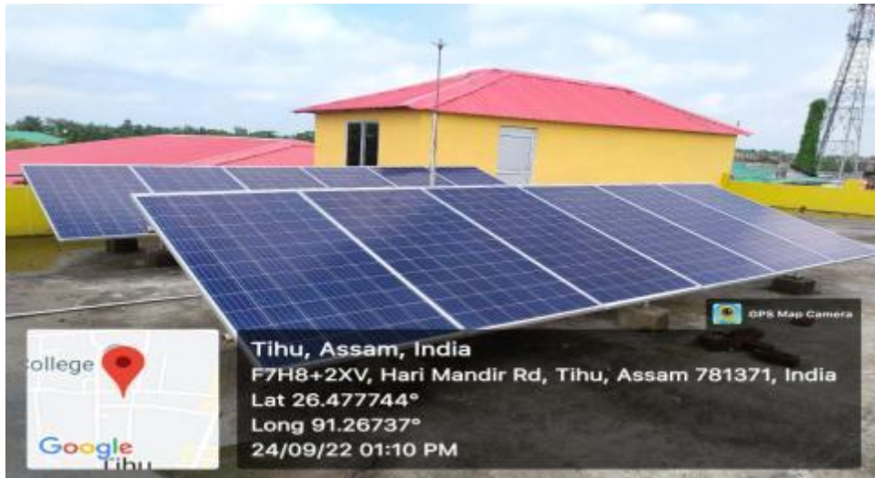
Photovoltaic Panels (Solar Panels)
