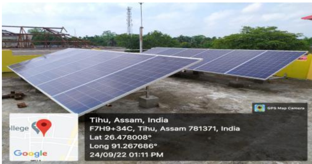
Photovoltaic Panels (Solar Panels)
